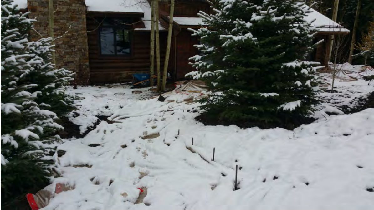
This photos depicts the new sidewalk from the new driveway to the existing house front door
