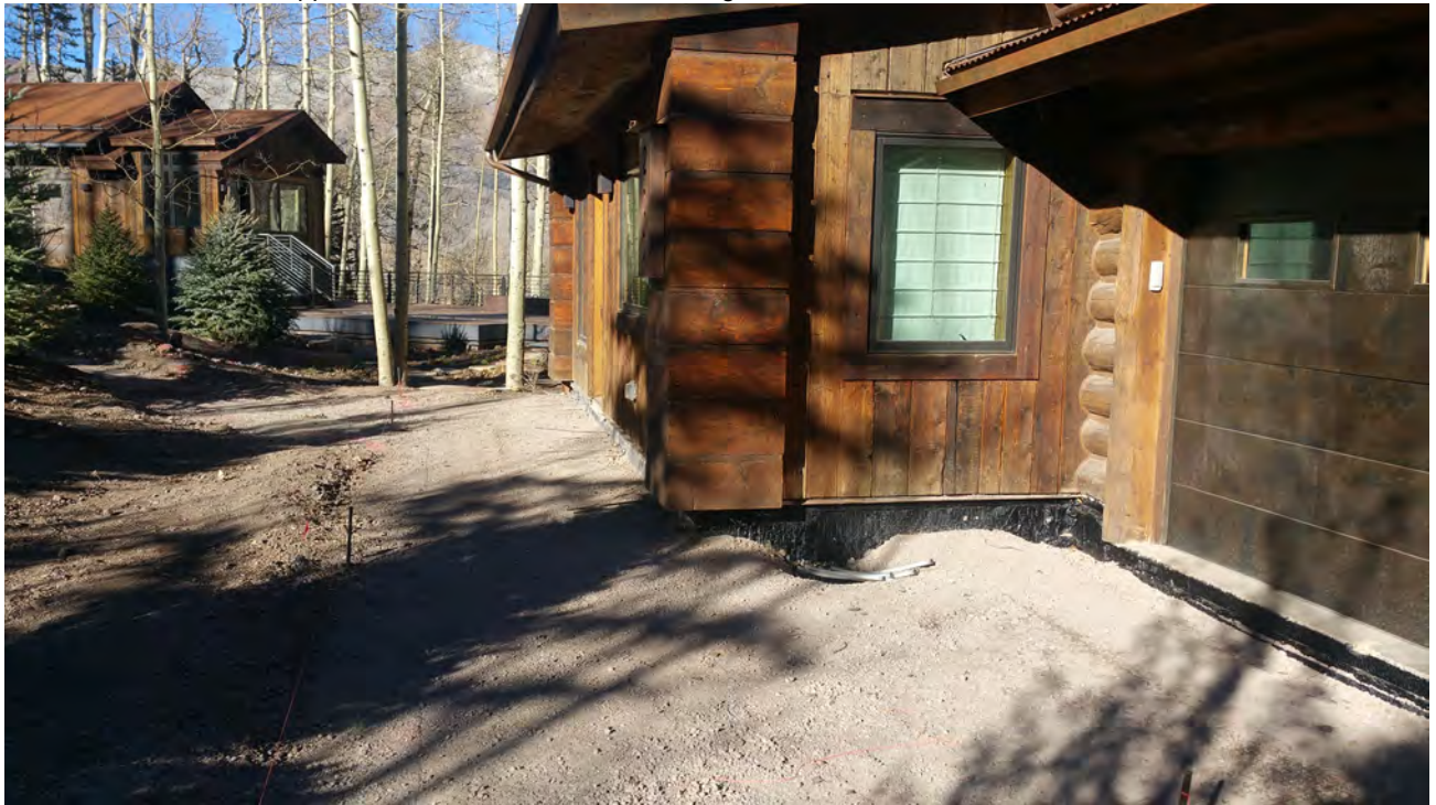
Existing 1 car garage door to be removed and replaced with one small door and window
