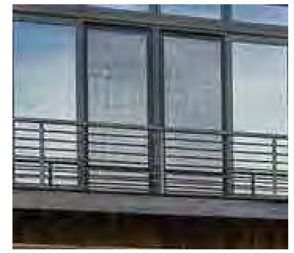
TYPICAL WINDOW CURTAIN WALL AND RAIL FINISH TO BE DARK BRONZE WITH STEEL HEADERS PER ELEVATIONS
