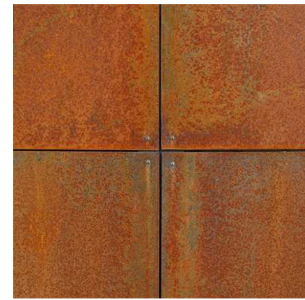
M1 RUSTED PANELS RUSTED
