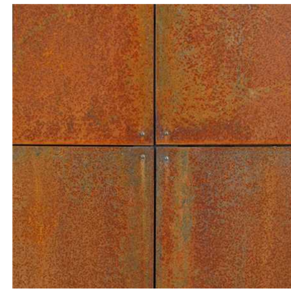
M1 RUSTED PANELS RUSTED
