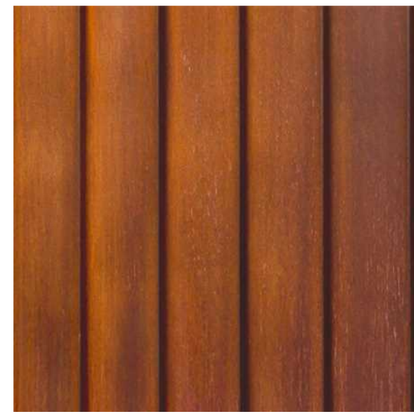
R1 STANDING SEAM ROOF RUSTED
