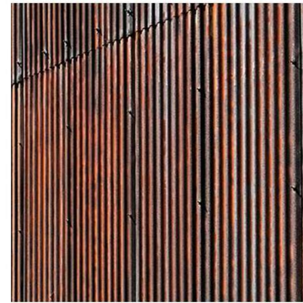
RUSTY CORRUGATED METAL SIDING
