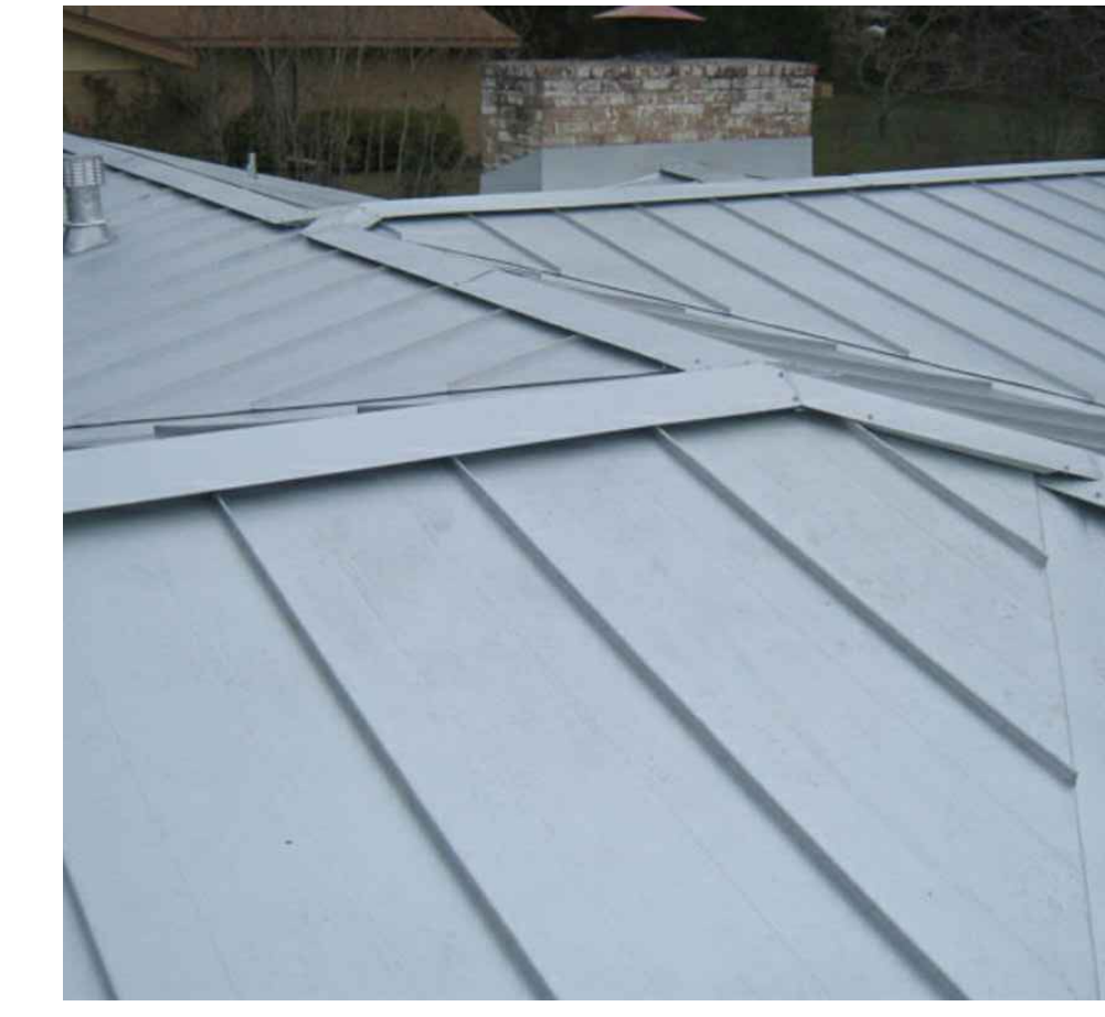
2" FIELD-LOK STANDING SEAM MTL ROOFING FINISH: WEATHERED ACRYLIC COATED GALVALUME MANUFACTURER: ATAS INTERNATIONAL
