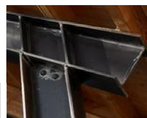
EXPOSED STEEL STRUCTURE
