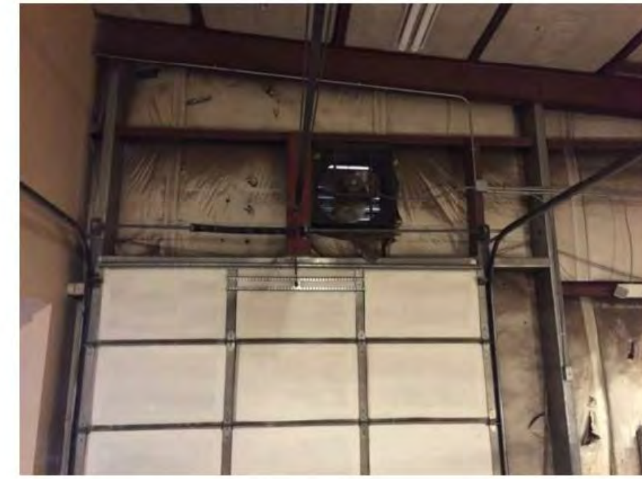
Photo #5: Repair Garage general exhaust fan
