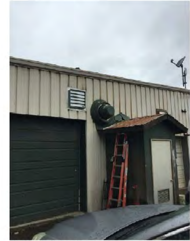
Photo #4: Repair Garage vehicle capture exhaust fan and general exhaust discharge
