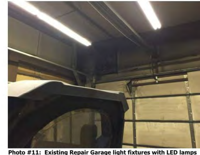
Photo #11: Existing Repair Garage light fixtures with LED lamps
