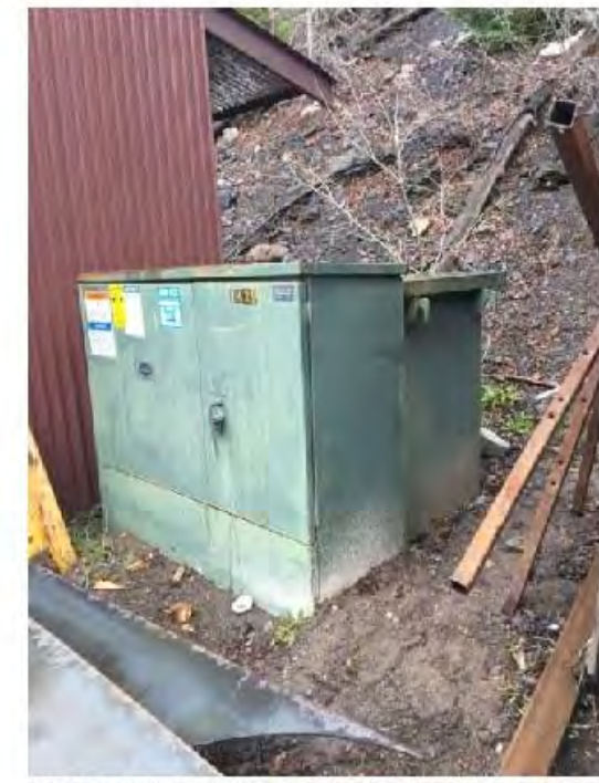
Photo #8: Existing exterior transformer and gear
