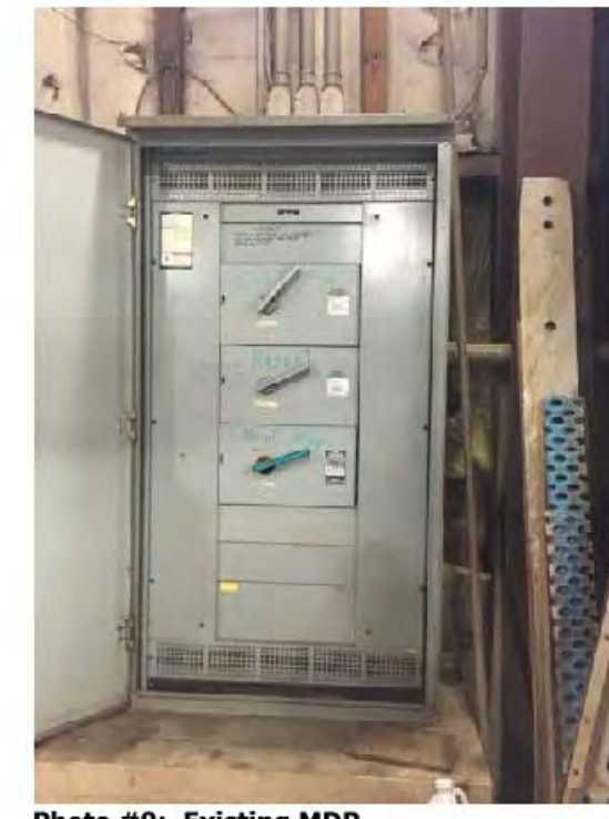
Photo #9: Existing MDP
