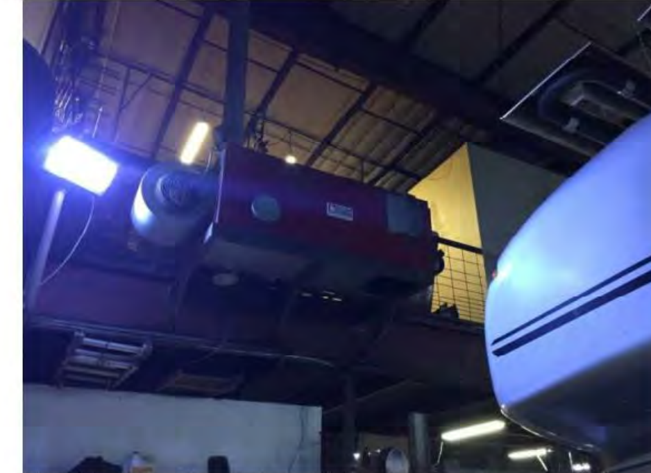
Photo #2: Waste oil heater located in Repair Garage that serves the Upper Level
