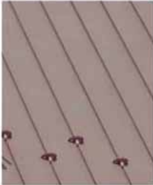
RUSTED STANDING SEAM METAL ROOF
