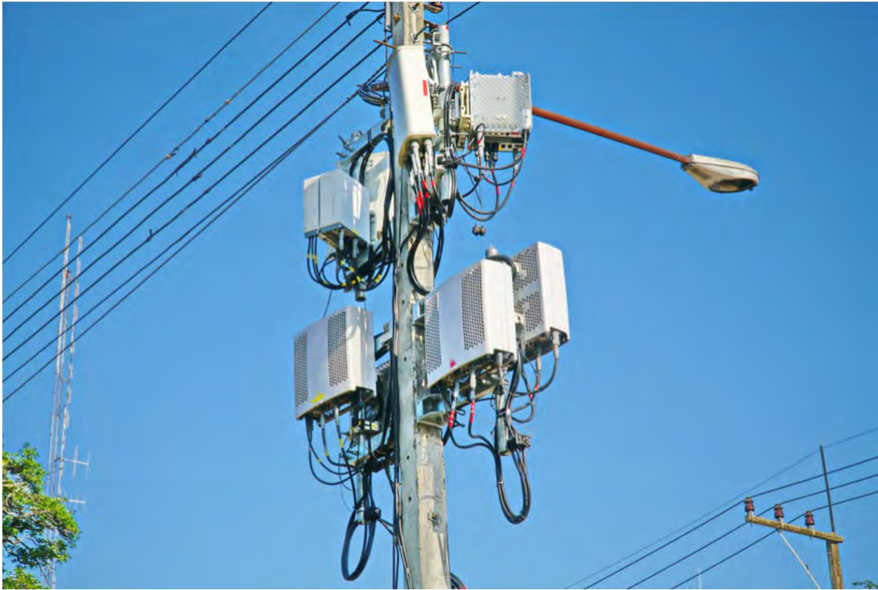
1) Multiple carriers mounted on exterior of existing pole
