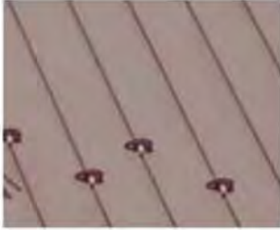
RUSTED STANDING SEAM METAL ROOF
