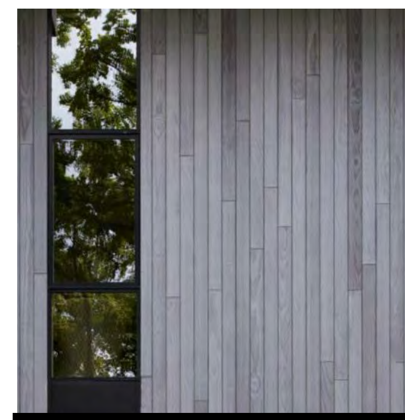
WOOD SIDING - SILVER PATINA NATURAL UNFINISHED WOOD MEANT TO PATINA TO A SILVER GREY FINISH. INSTALLED IN VERTICAL PATTERN USING 4-6" WIDE BOARDS
