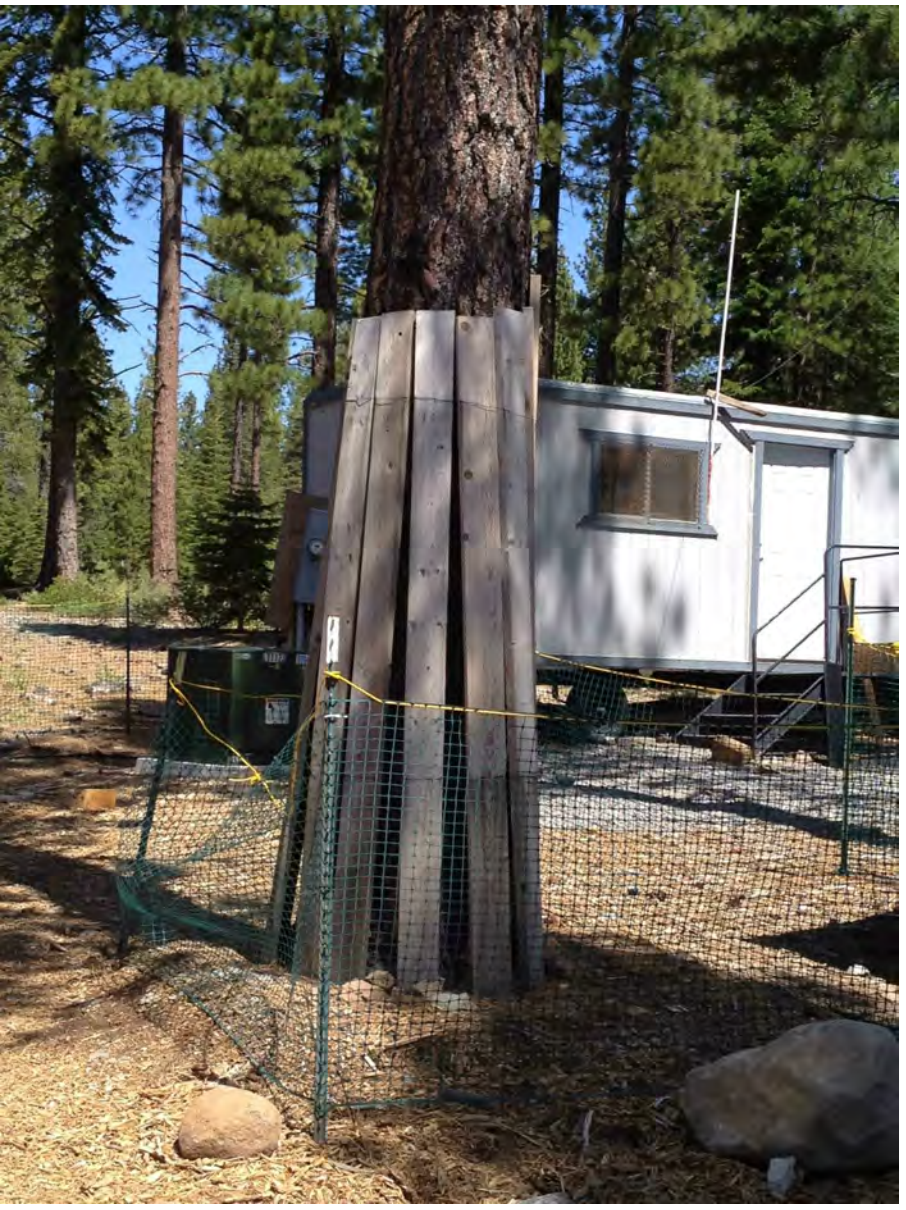
ILLUSTRATION OF TREE PROTECTION. NOTE: ALL TREES TO REMAIN WITHIN THE LIMITS OF CONSTRUCTION SHALL BE PROTECTED AS ILLUSTRATED ABOVE.
