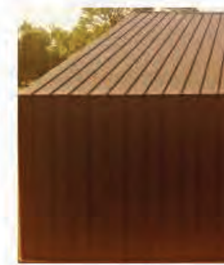
STANDING SEAM RUSTED METAL ROOF AND SIDING
