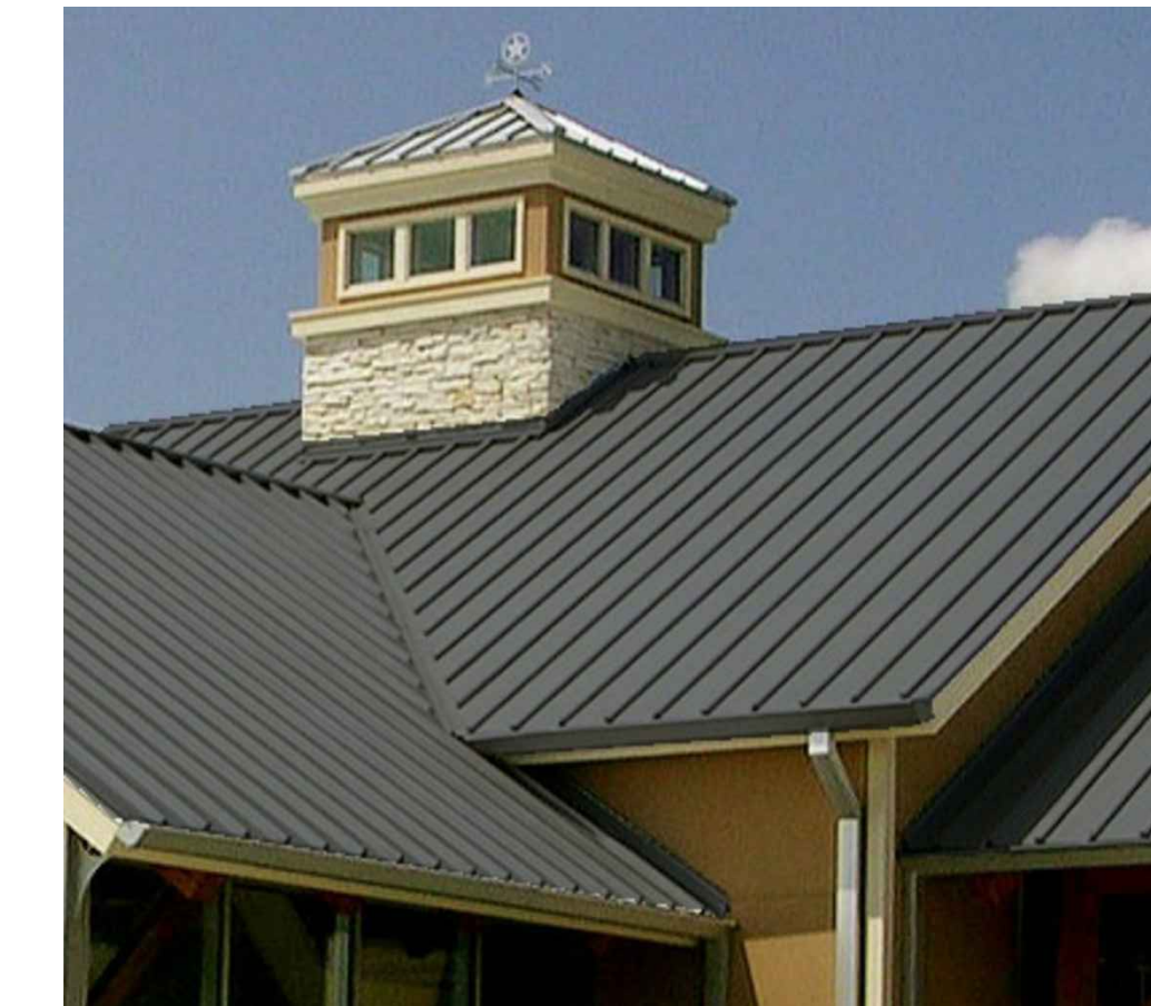
2" SNAP LOCK STANDING SEAM MTL ROOFING FINISH: MUSKET GRAY MANUFACTURER: DREXTEL METALS
