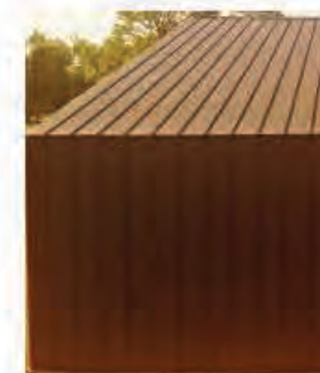
STANDING SEAM RUSTED METAL ROOF AND SIDING
