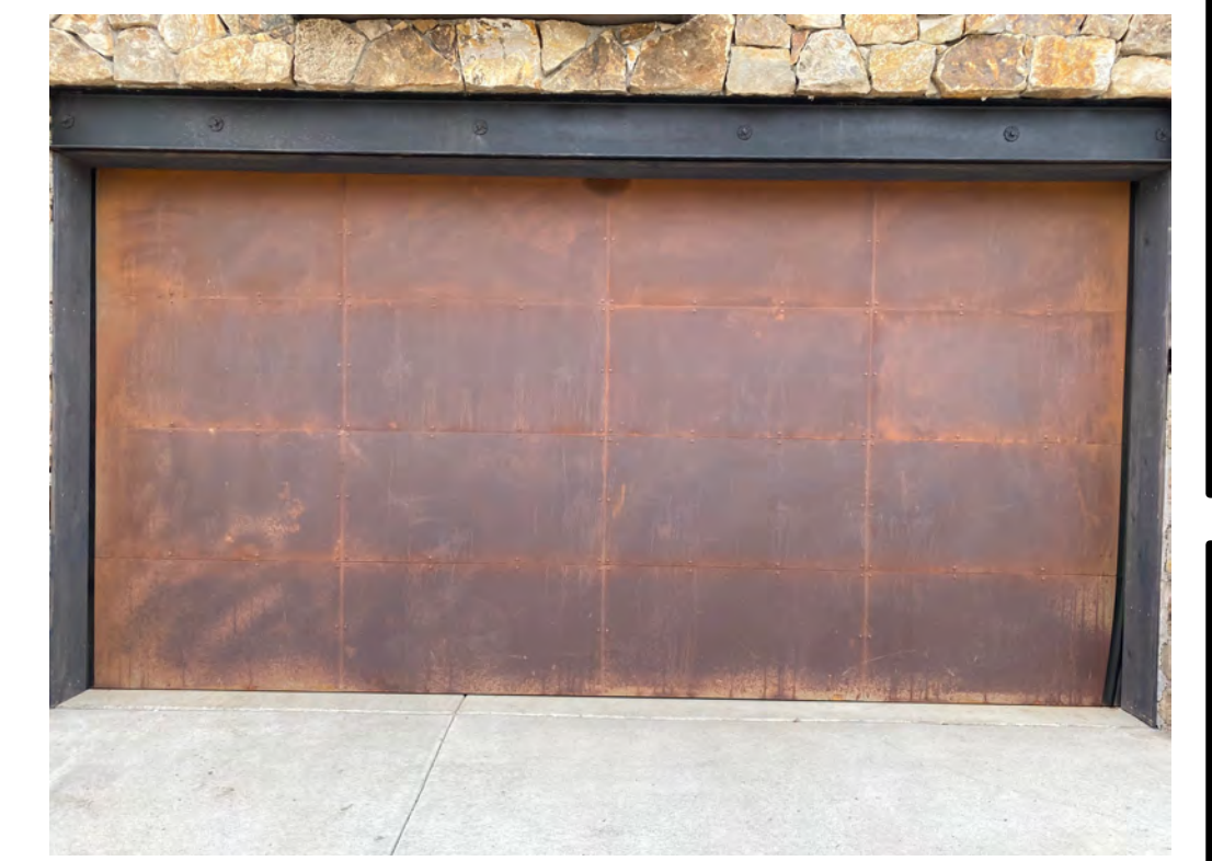
Garage door rusted metal flat 2'x4'
