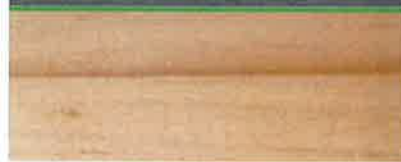
Pella's casement window after 7 months of exposure to moisture.*
