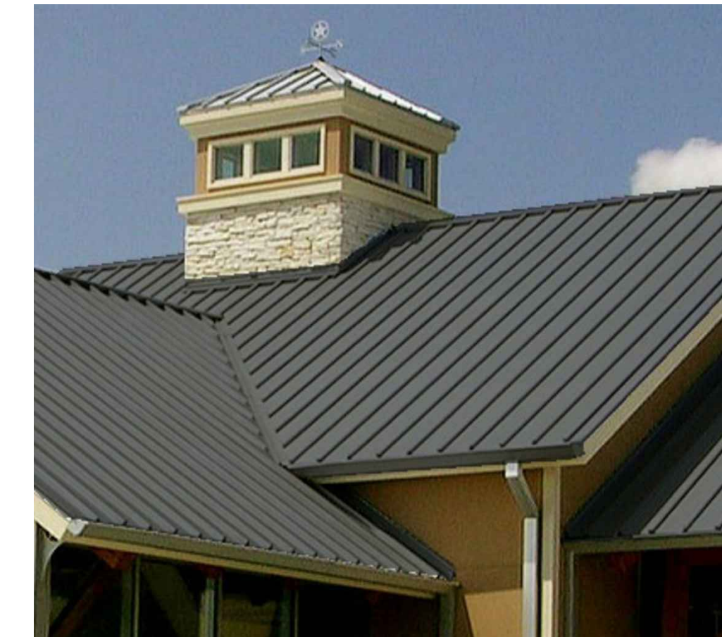
2" SNAP LOCK STANDING SEAM MTL ROOFING FINISH: MUSKET GRAY MANUFACTURER: DREXEL METALS
