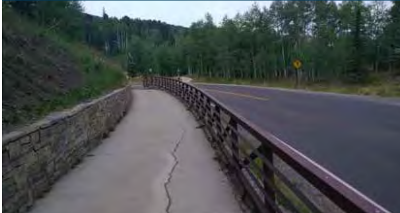
Boulevard Trail East is a shared use path that is also considered a sidepath because it is adjacent to Mountain Village Blvd.
