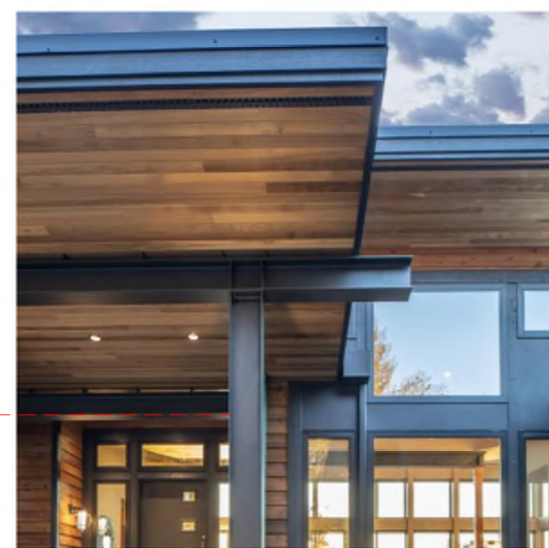
STEEL STRUCTURE: EXPOSED WIDE FLANGE STEEL, DARKING BLUING FINISH OR OIL RUB
