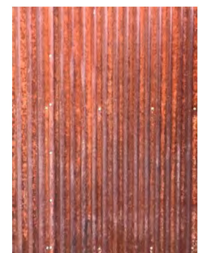
RUSTED CORRUGATED SIDING
