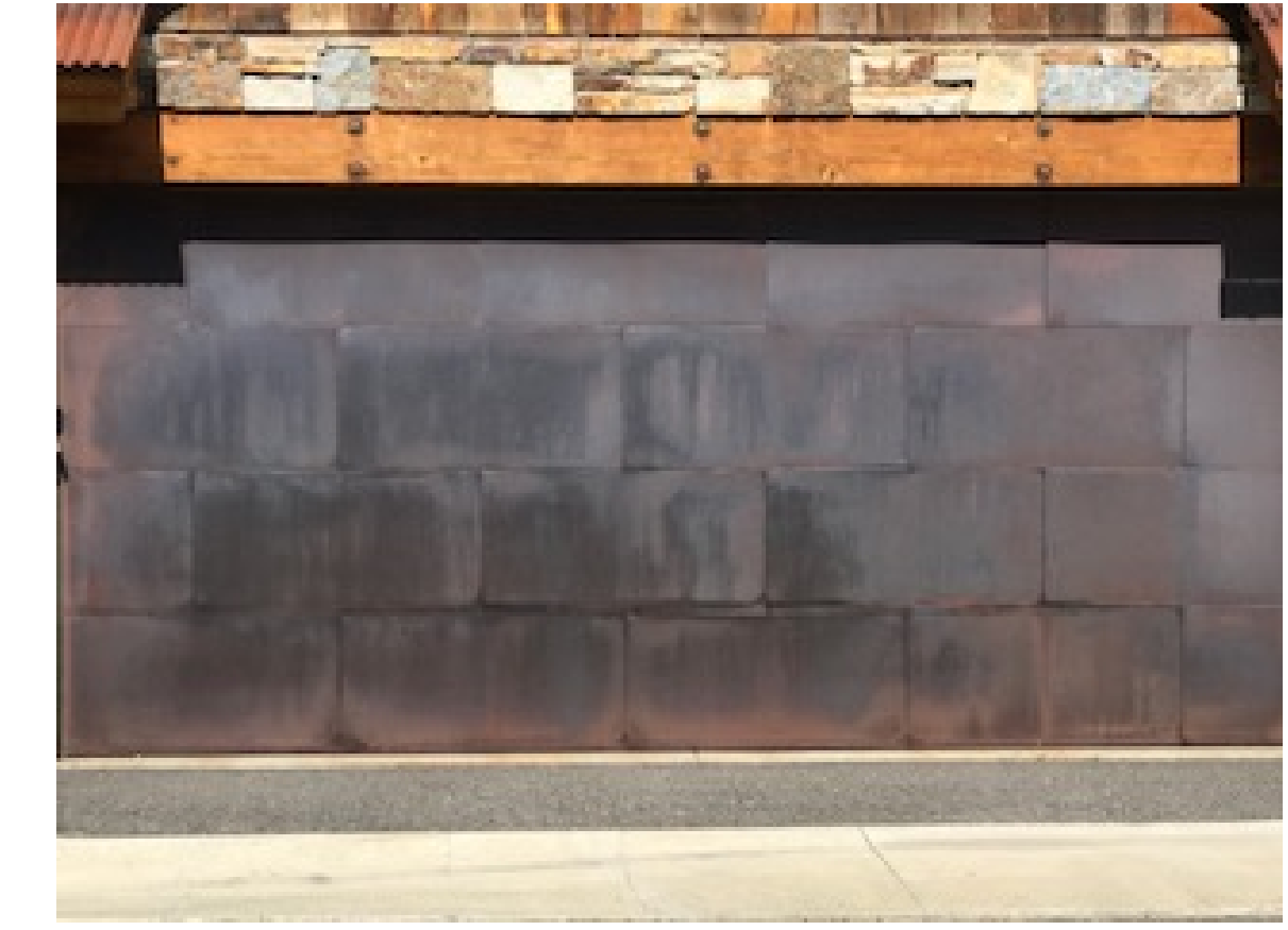
RUSTED 24x48 METAL PANELS
