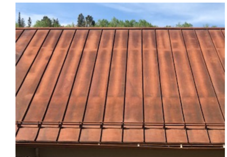
RUSTED STANDING SEAM ROOFING
