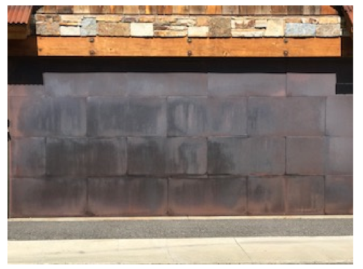
RUSTED 24x48 METAL PANELS
