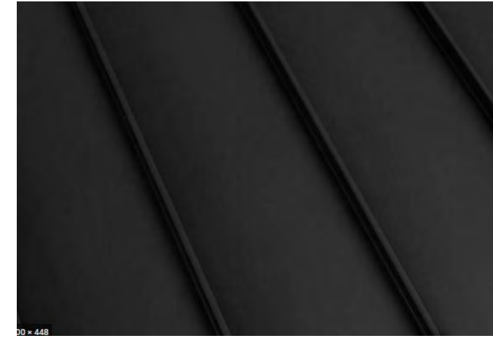
DARK PREFINISHED METAL ROOF WILL BE EITHER A DARK STEEL OR DARK BROWN PATINA FINISH PER 17.5.6.C.3.C.iv
