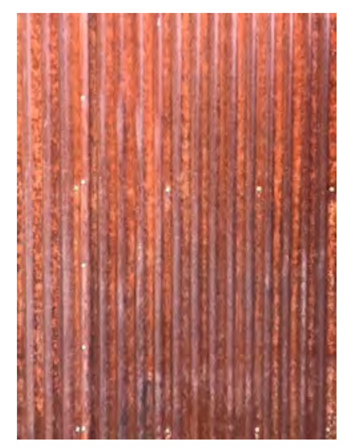
RUSTED CORRUGATED SIDING
