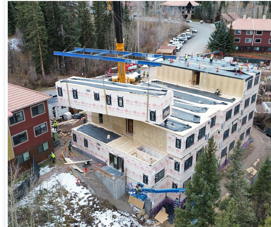
The modulars for the east building of Village Court Apartments Phase IV were set in November.
